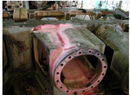
Removing & Inserting Complete Top Section Due To Cracks
